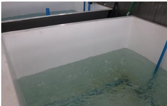
One of the segmented water tanks
